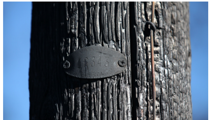
A Garkane pole charred from the Mangum fire in 2020
